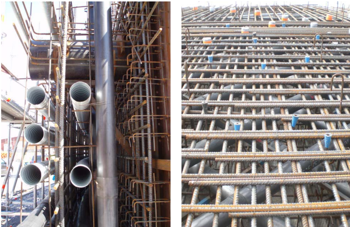
Figure 2. Prestressing duct and reinforcement arrangement in cylinder and dome part of EPR TM .
